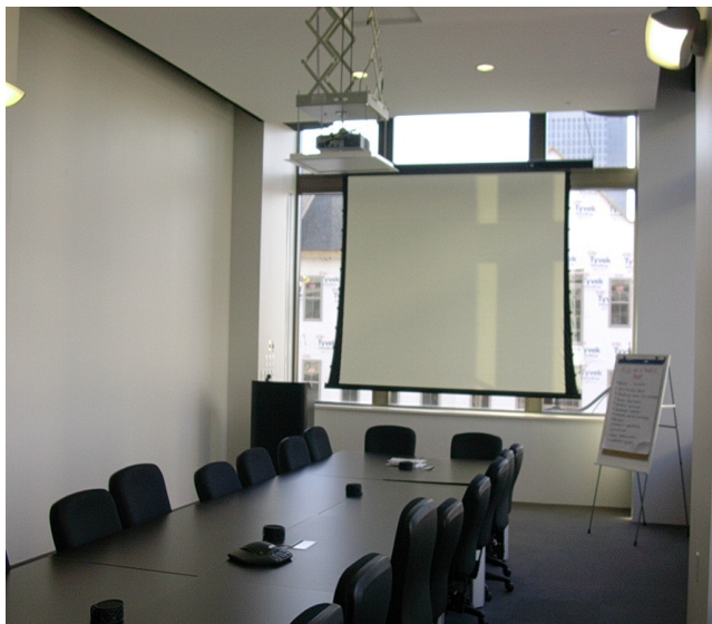
To give the Chamber a clean, finished look in its board room, IBS installed a ceiling-recessed lift system for the projector. IBS also set up the wireless conference phone shown on the table.
